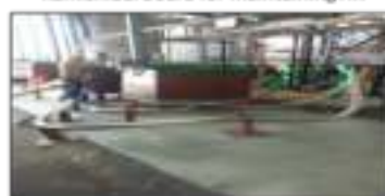
Hanging of Flexible pipes for ease of cleaning
